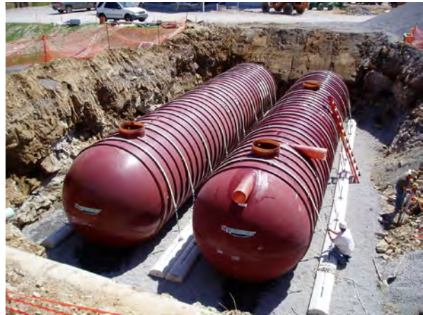
Figure 12: Underground water storage tank
