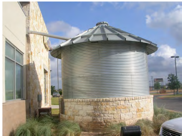
Figure 13: Decorative above ground rainwater catchment tank
